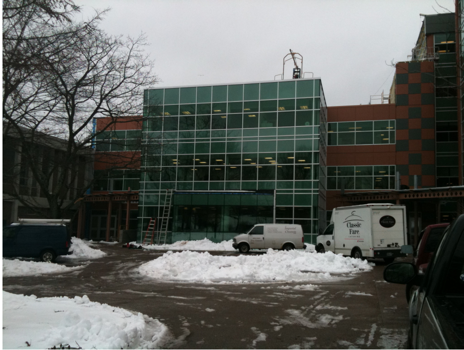
Figure 5: The Atrium Building as seen from Inglis Street. The ICA & the Department of Astronomy & Physics share the top floor.
